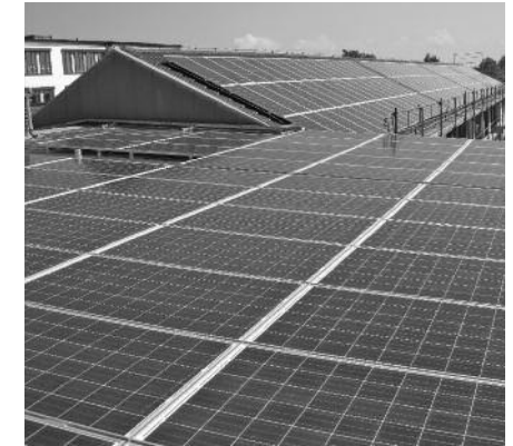
Photovoltaik in Bürgerhand in Eching
